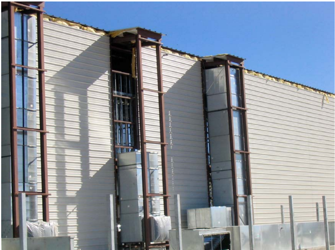
HVAC duct enclosures
