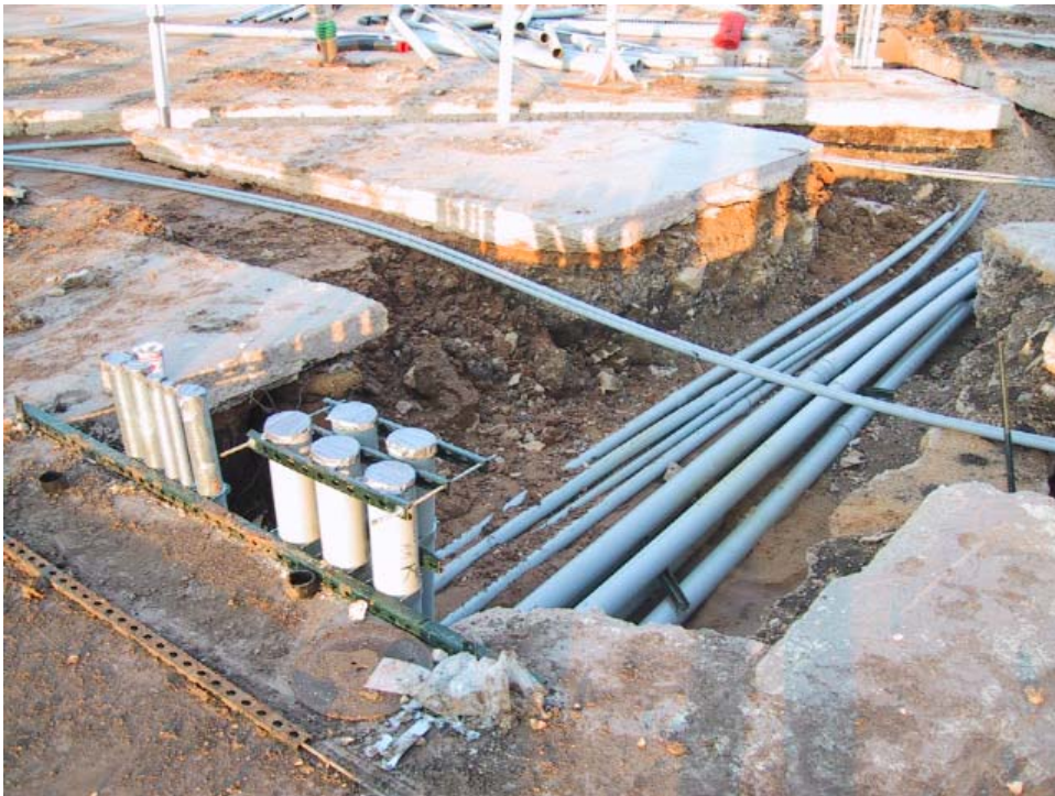
Electrical power stubbed into mechanical room
