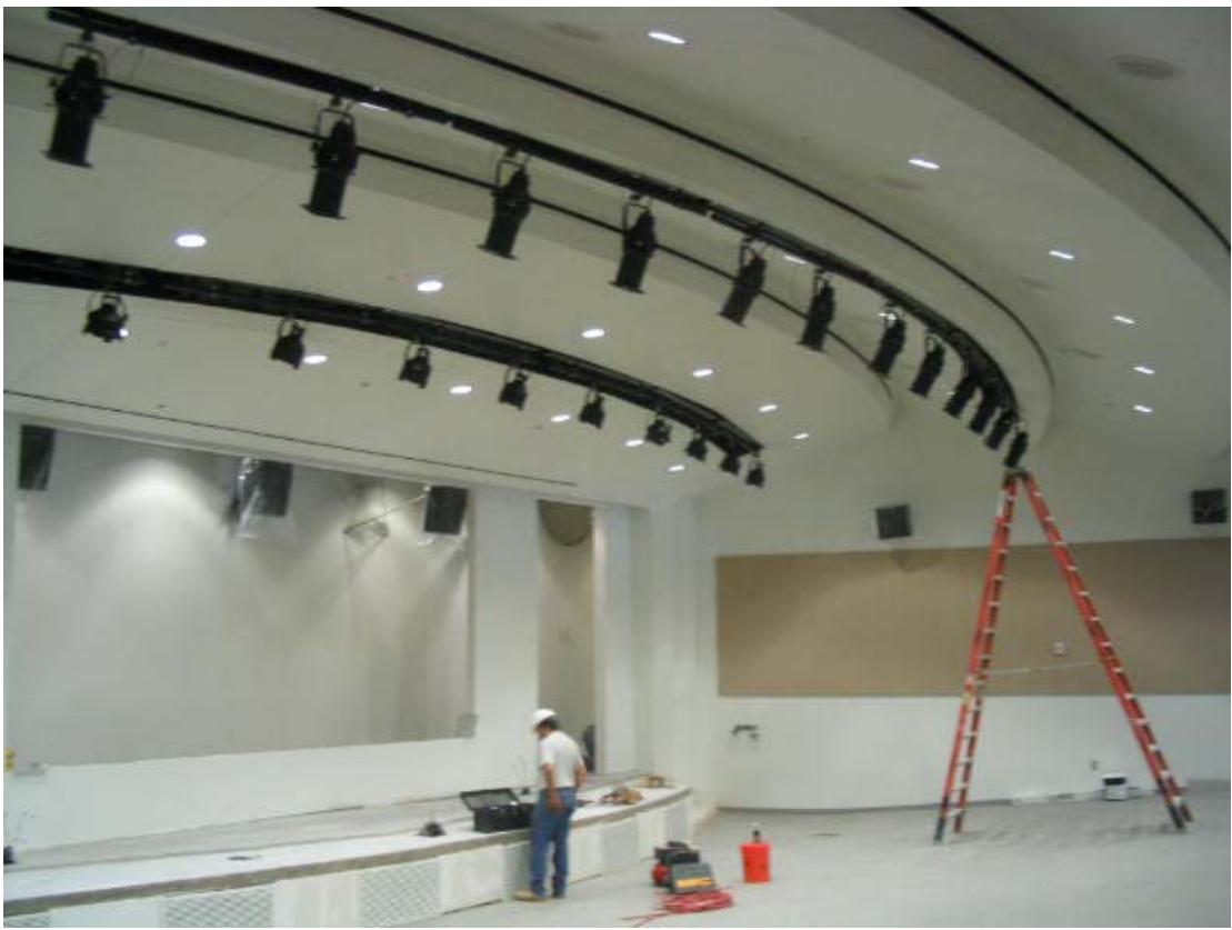
Auditorium lighting installed
