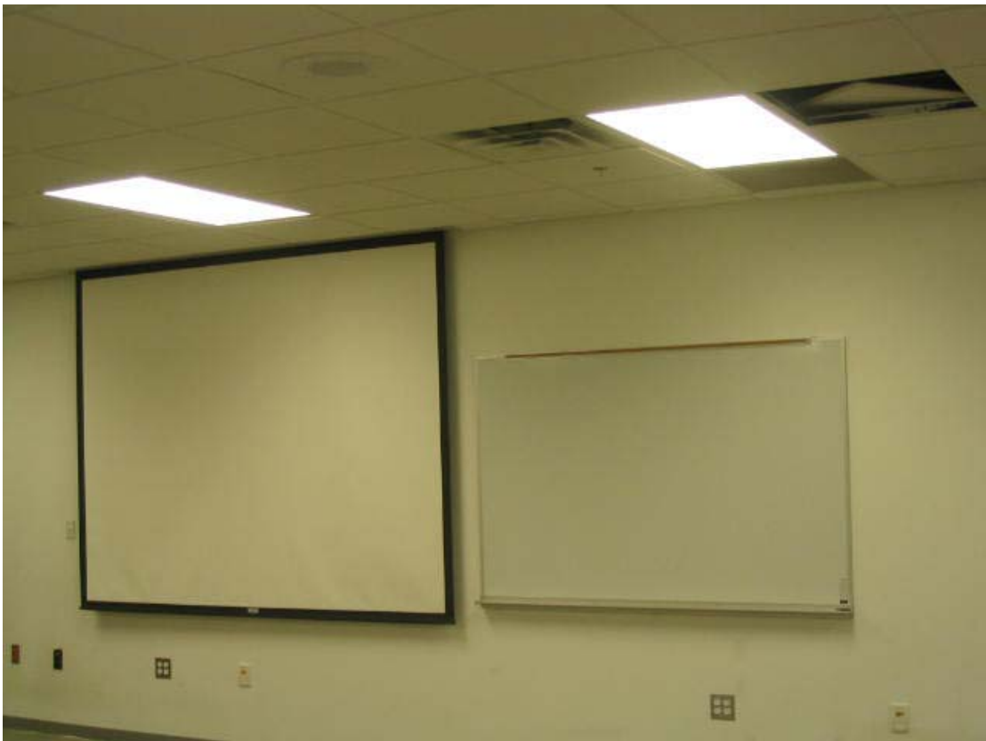
Classroom projection screen and whiteboard installed
