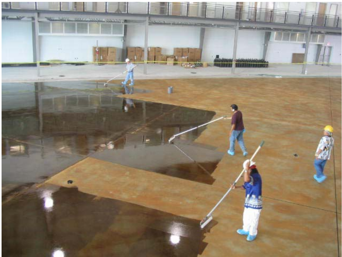
Concrete staining of main hall
