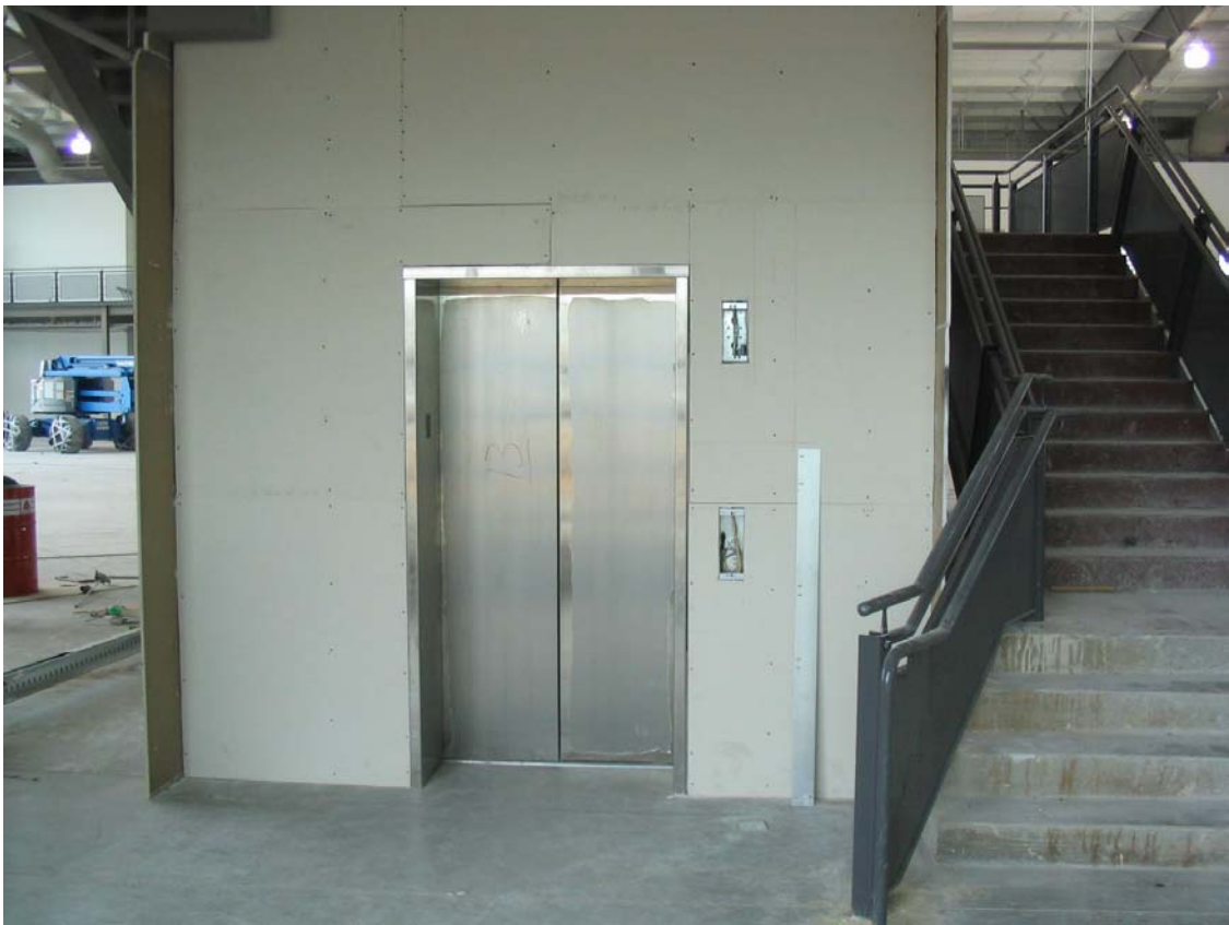
Elevators being readied
