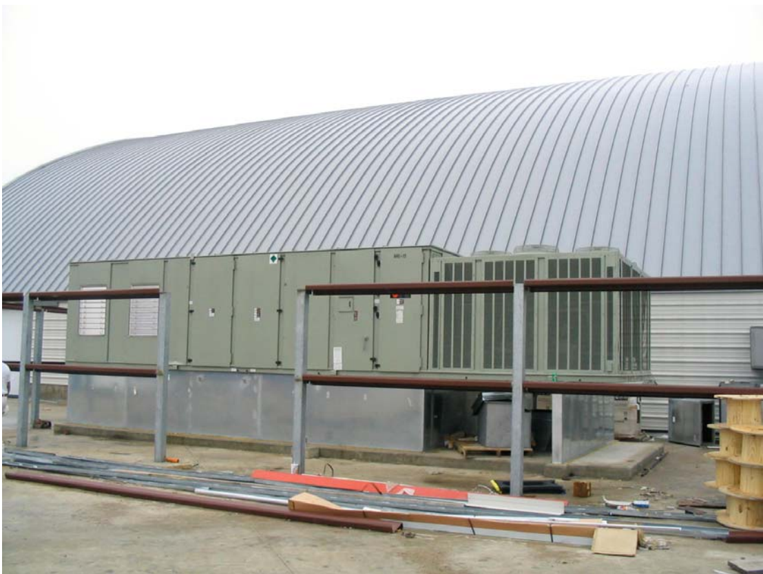
Building B mechanical installed
