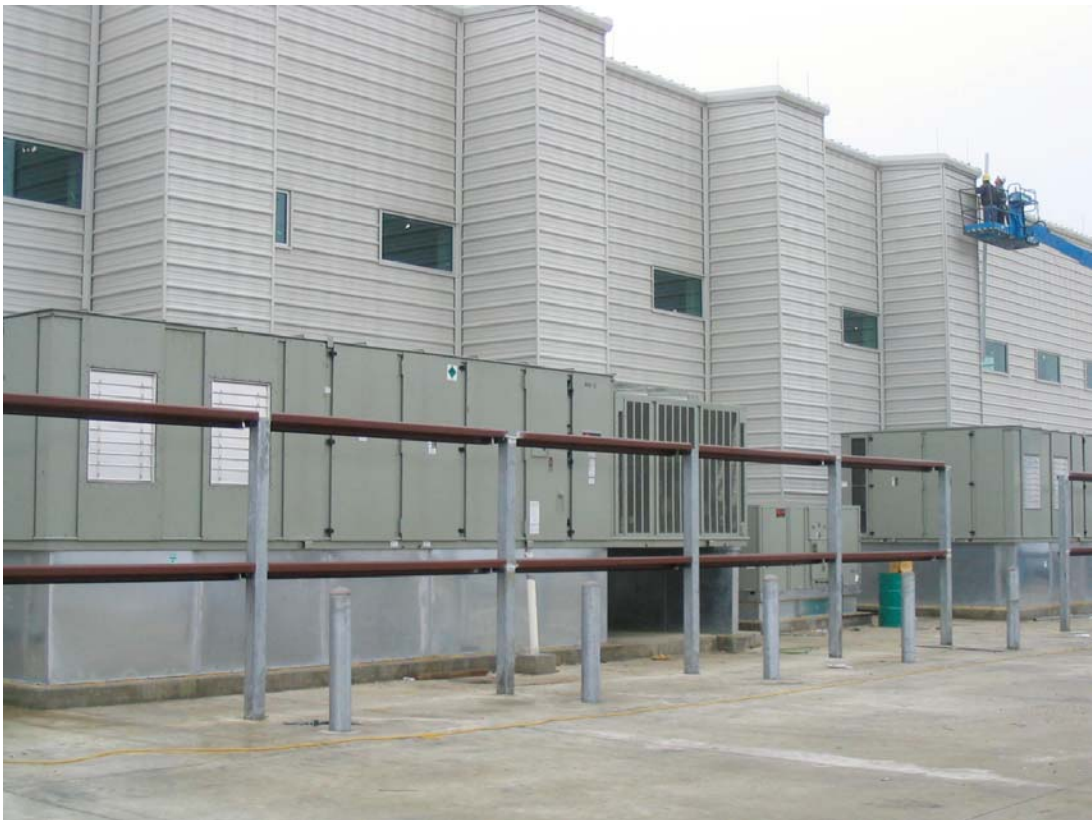
Building A mechanical installed
